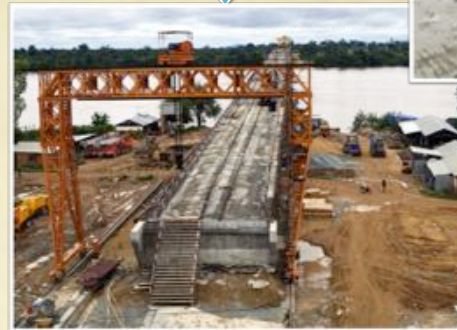
The Sekong Bridge, a $20 million project financed with Chinese aid money. Retrieved April 25, 2013, from http://www.nytimes.com/slideshow/2006/09/17/world/20060918_CHINA_SLIDESHOW_2.html
