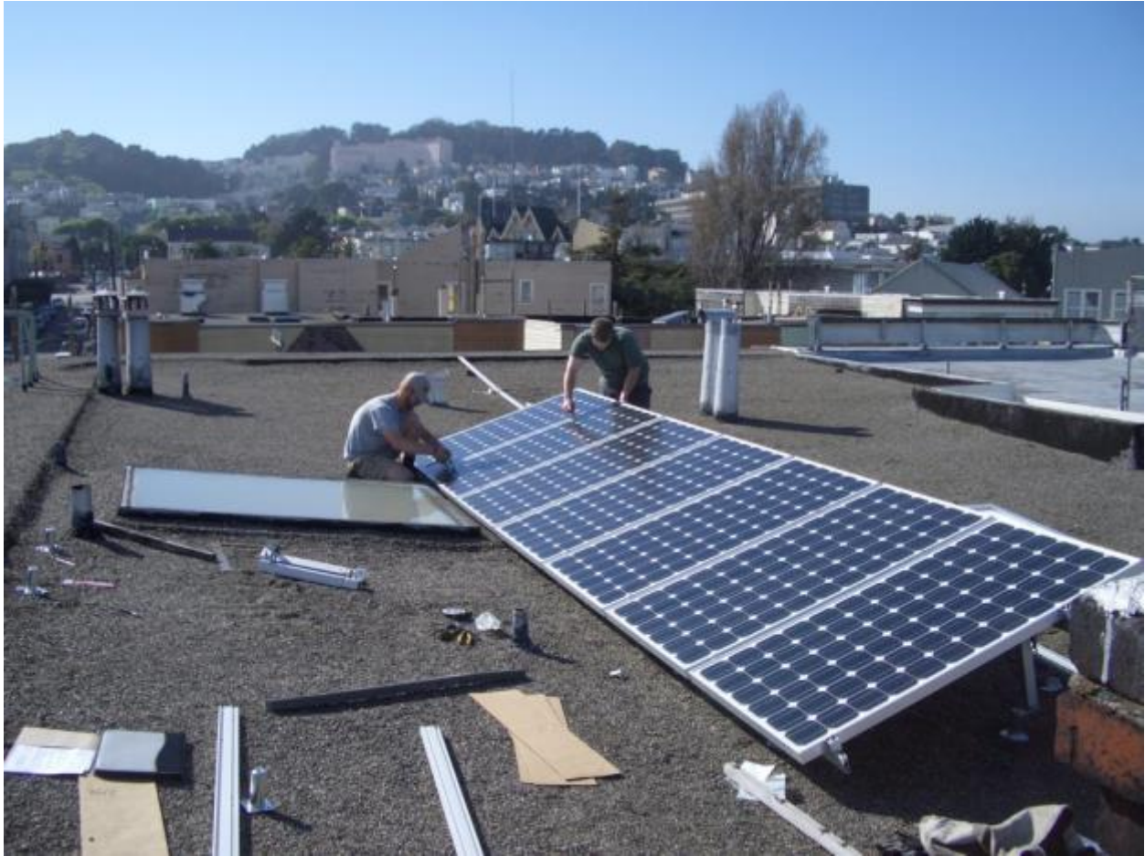
Installing Photovoltaics on the Sally McCracken Building (Image from Lewis & Clark Digital Scholarship Multisite: Oregon Solar Policy)
